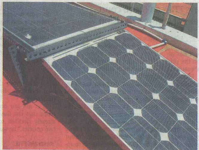
The company has started a rooftop solar power project in Chandigarh and is carrying out EPC works for its sister company Punj Lloyd Solar.
